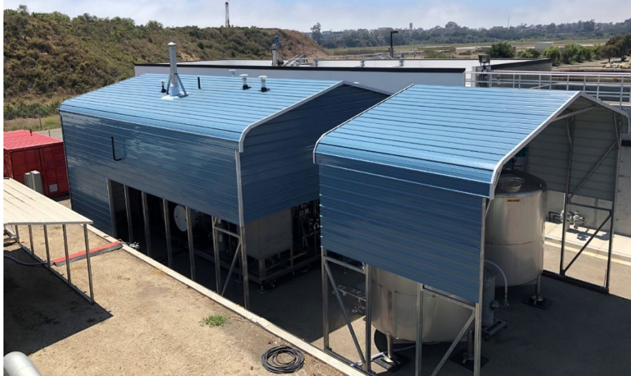
Figure 5: Covered Processing Equipment
