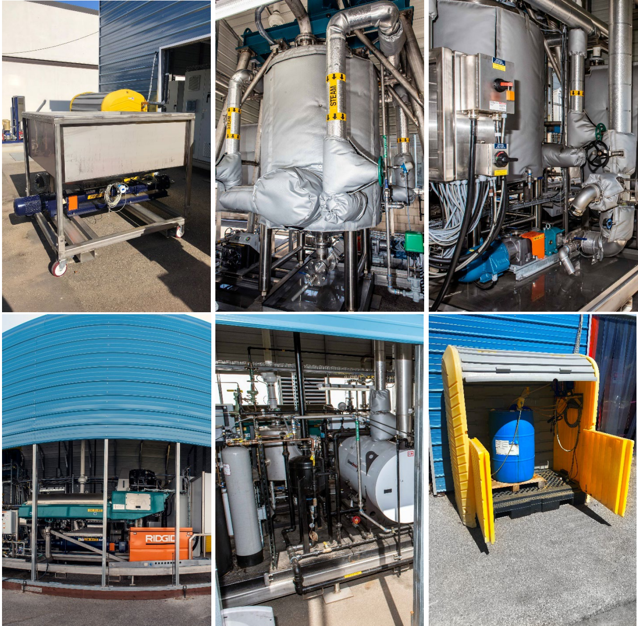
Figure 7: Lystek THP Equipment
